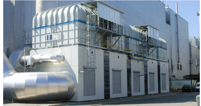
Incineration installation for thermal regenerative flue air purification
