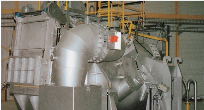
Aluminium tank furnace
