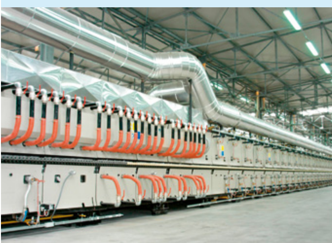
Roller hearth furnace
